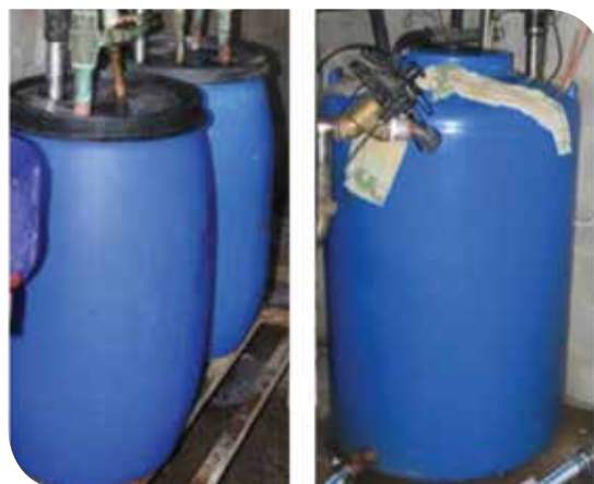
Figure 6 Examples of different types of wash tanks
