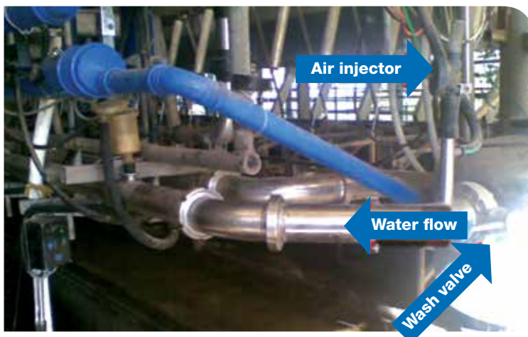
Figure 10 Air injector and wash valve on a looped milk line (example only)
