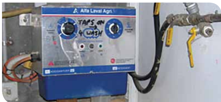
Figure 5 A semi-automatic wash controller for a bulk milk vat (example only)
