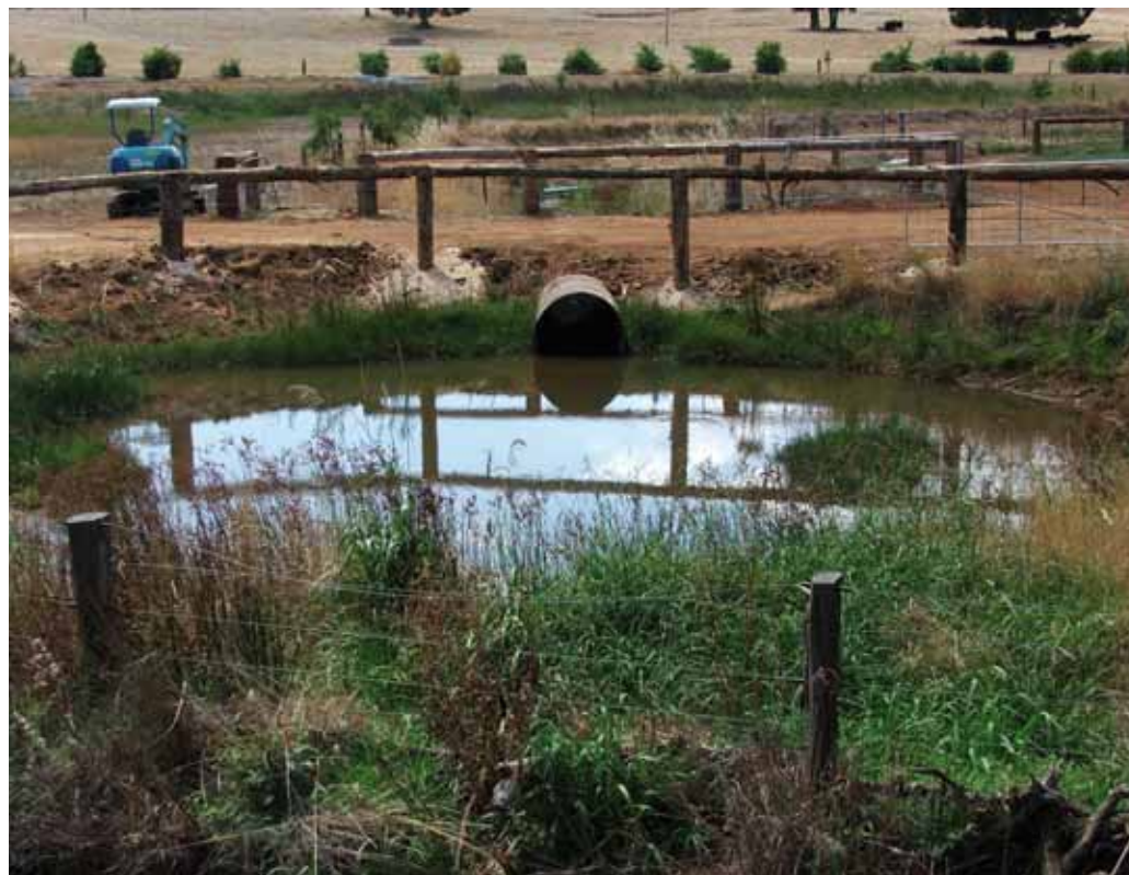
Figure 4.3 A sedimentation settling basin constructed at the end of a main drain.
