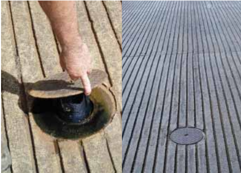
Pop-up portals used to flood wash yards at the Bell Dairy
