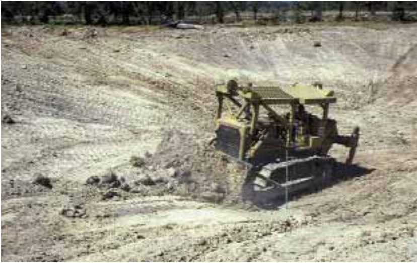
A dozer being used to build the effluent pond at the Gulberti dairy near Busselton
