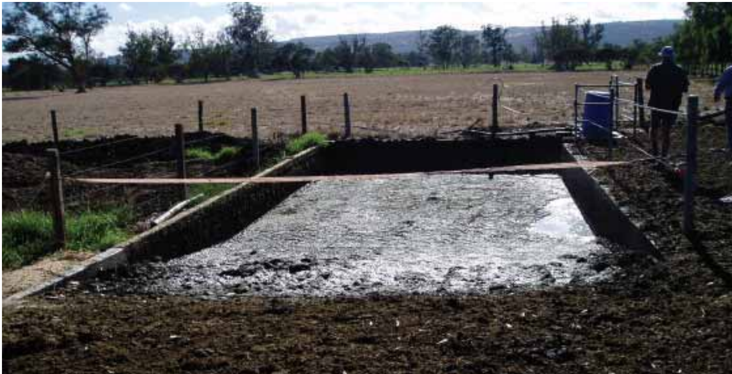
Newly constructed effluent bunker with adjoining trafficable sump at Piggott dairy in Harvey
