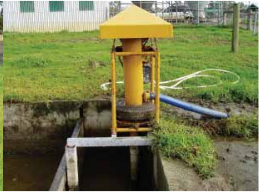
The Rankin pump is a favoured choice because of its simple design and robust performance
