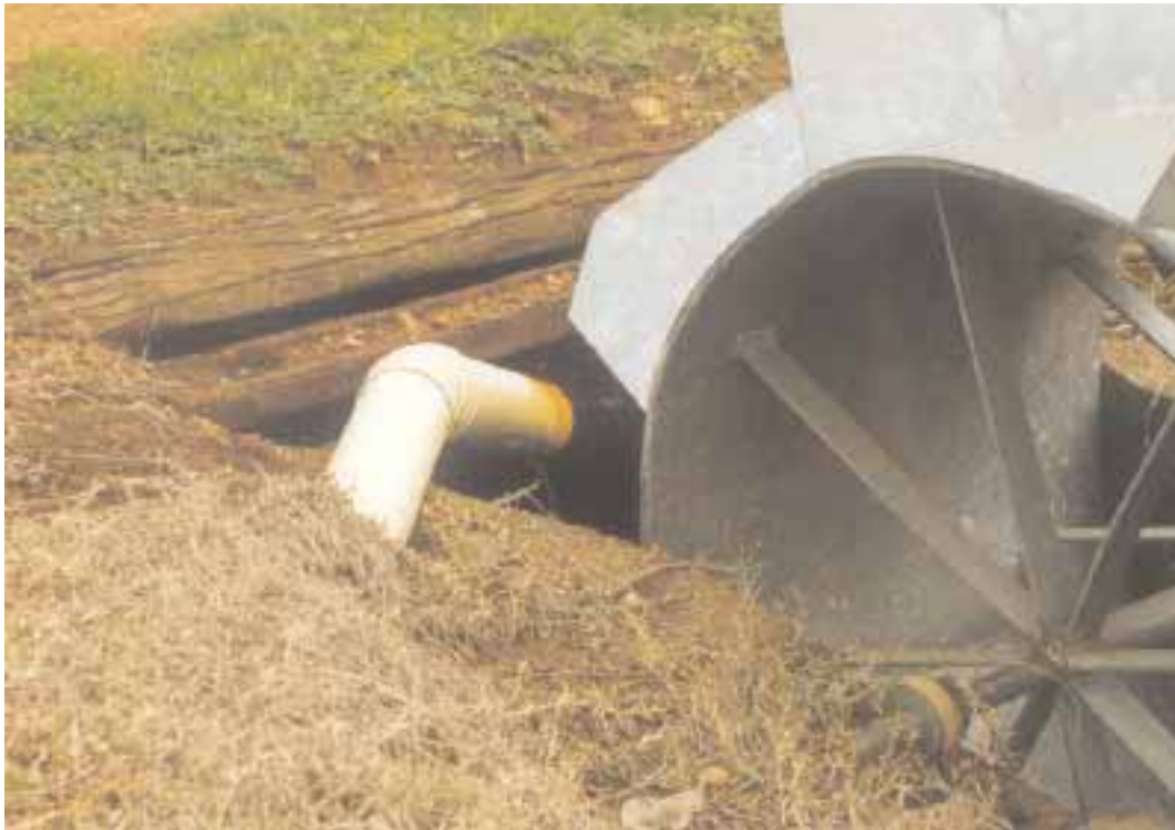
Effluent pipe discharging directly into flood irrigation channel
