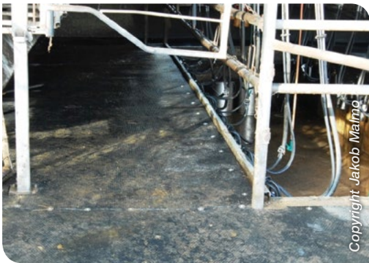
Rubber matting may be strategically placed in high traffic areas such as entrance and exits of the bails where cows are likely to twist and turn.
