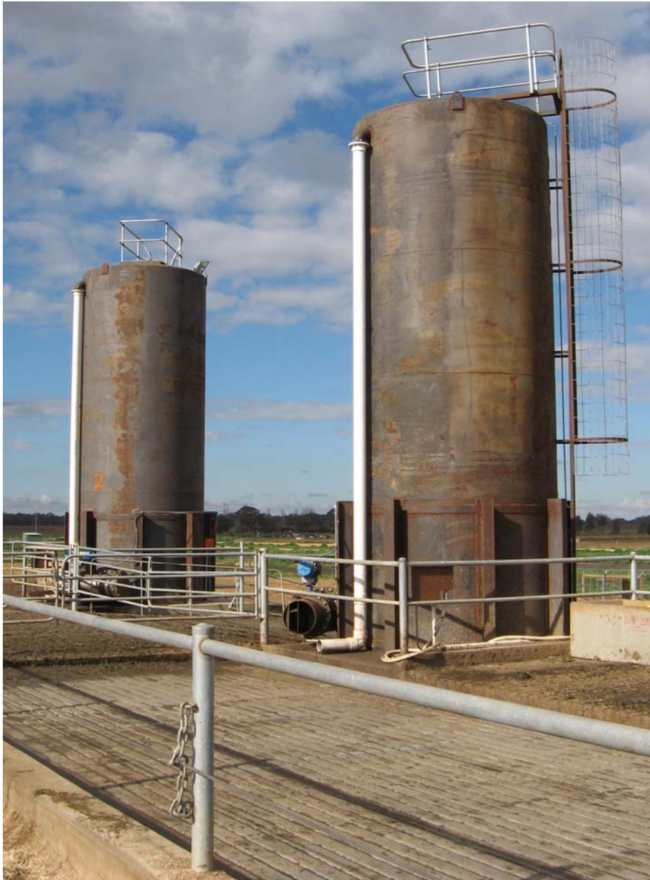
Figure 1. Floodwash tanks and above-the-surface delivery for feedpad flushing.
