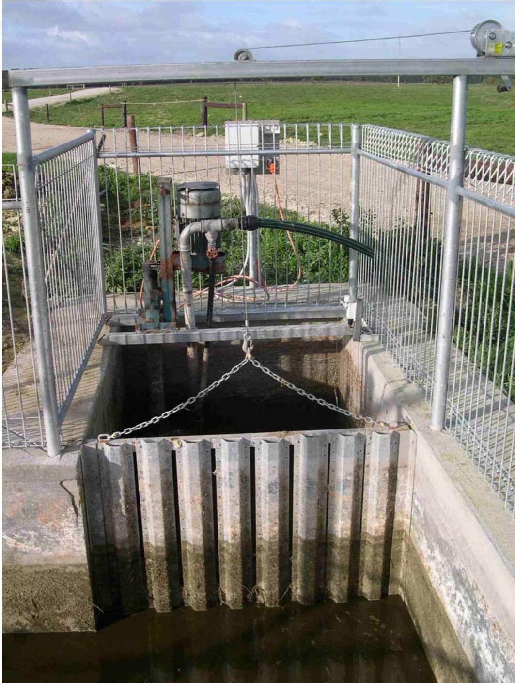
Figure 1. Vertical weir in trafficable solids traps (courtesy of Rural Solutions SA).
