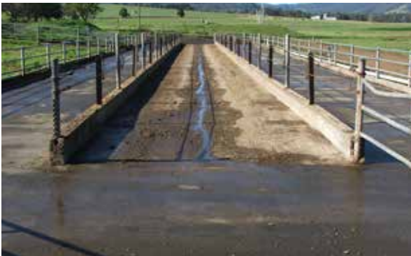
PMR fed out on fully concreted feedpad with nib wall, central feed alley
