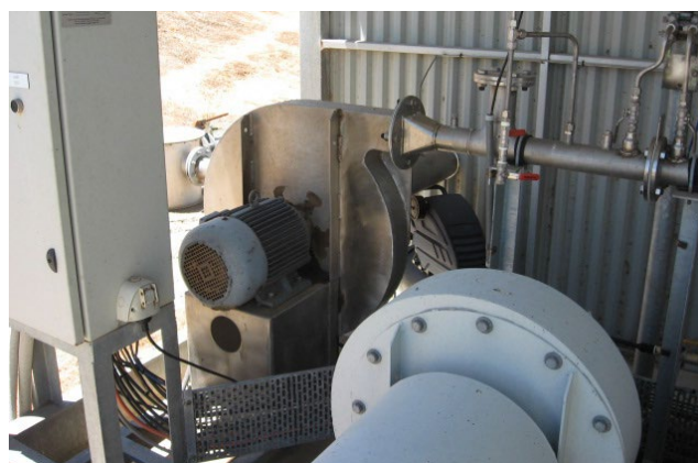
Biogas blower and flow meter. Photo courtesy of GWF Bears Lagoon Piggery
