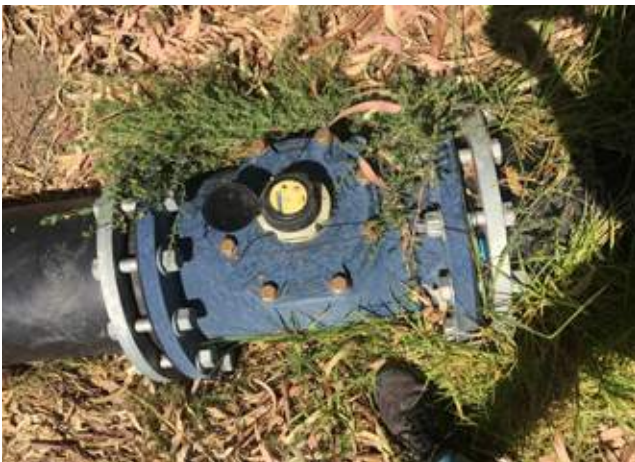
Figure 28 A paddlewheel meter installed in the field.
