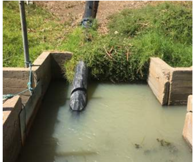
Figure 29 A paddlewheel meter installed in the field.
