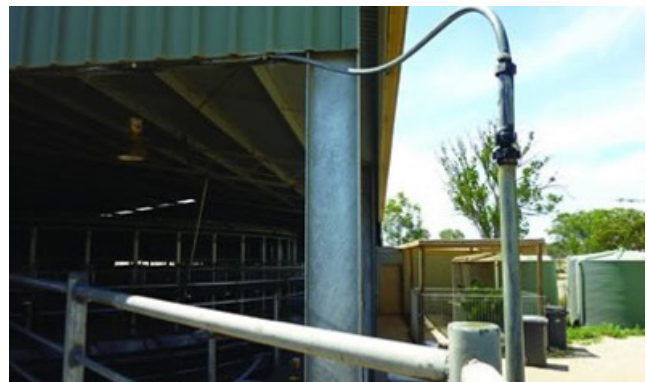
Spray curtain water supply and filter
