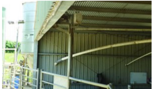
Polyethylene pipe attached to the dairy shed roof for the spray curtain
