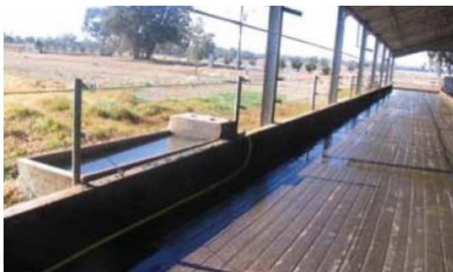
Note the position of water trough, grooving to help prevent cows slipping, water runoff from the roof to lane, high eaves and pitched roof to facilitate ventilation. The shed run north to south to use sunlight to dry cow standing areas
