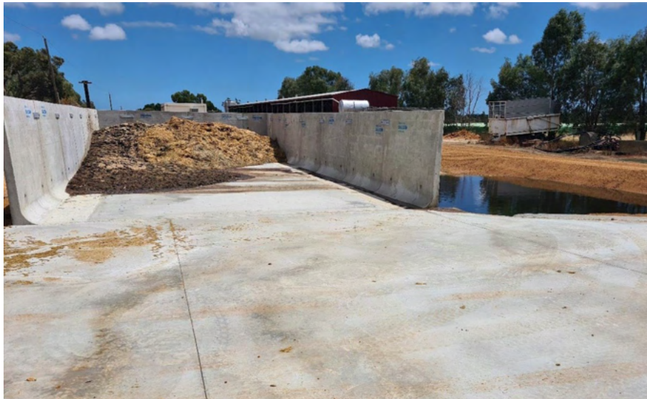
Solids storage pad with stormwater pond
